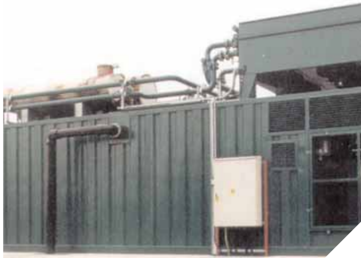
Landfill gas engine
